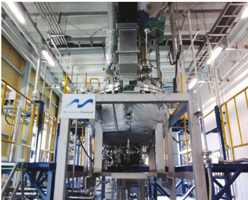
Figure 1: The newly completed demonstration facility
